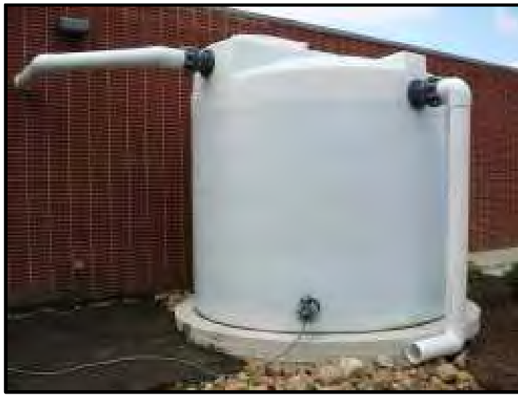
Photo 5-20. Rainwater Harvesting Storage Element
