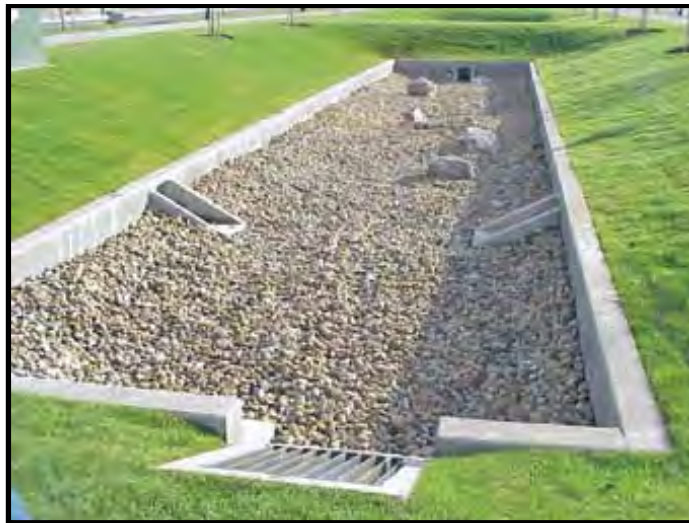
Photo 2-30. Surface Sand Filter (Source: City of Portland, OR)
