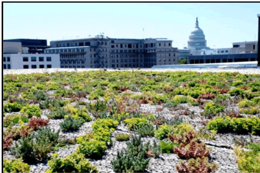
Photo 5-23. Green Roof – Washington, DC (Source: Healthy Roofs for Healthy Cities (Photo by US DOT))
