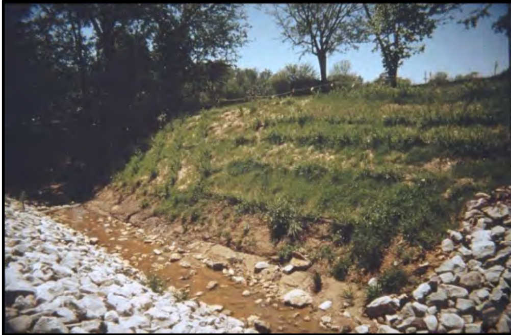
Photo 2-34. Eroded Streambank (Source: FISRWG, 1998)
