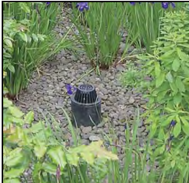
Photo 5-6. An Overflow within Bioretention
