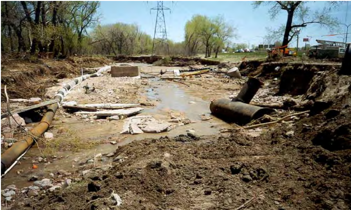
Photo 1-3. Pipeline damage in Colorado Springs.
