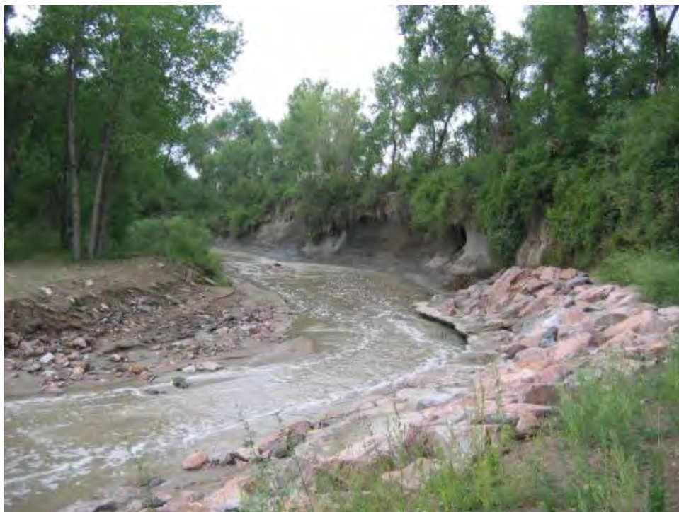
Photo 2-9. Monument Creek near Templeton Gap Floodway confluence Downstream view of showing channel degradation and riprap on eroding right bank (0133)
