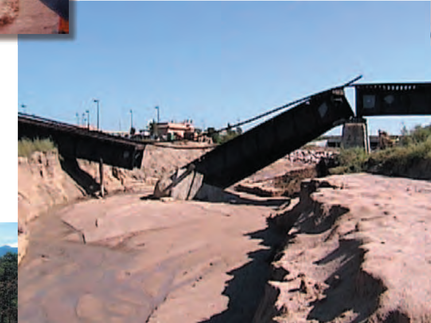
Failed Railroad Bridge, Sand Creek 2004
