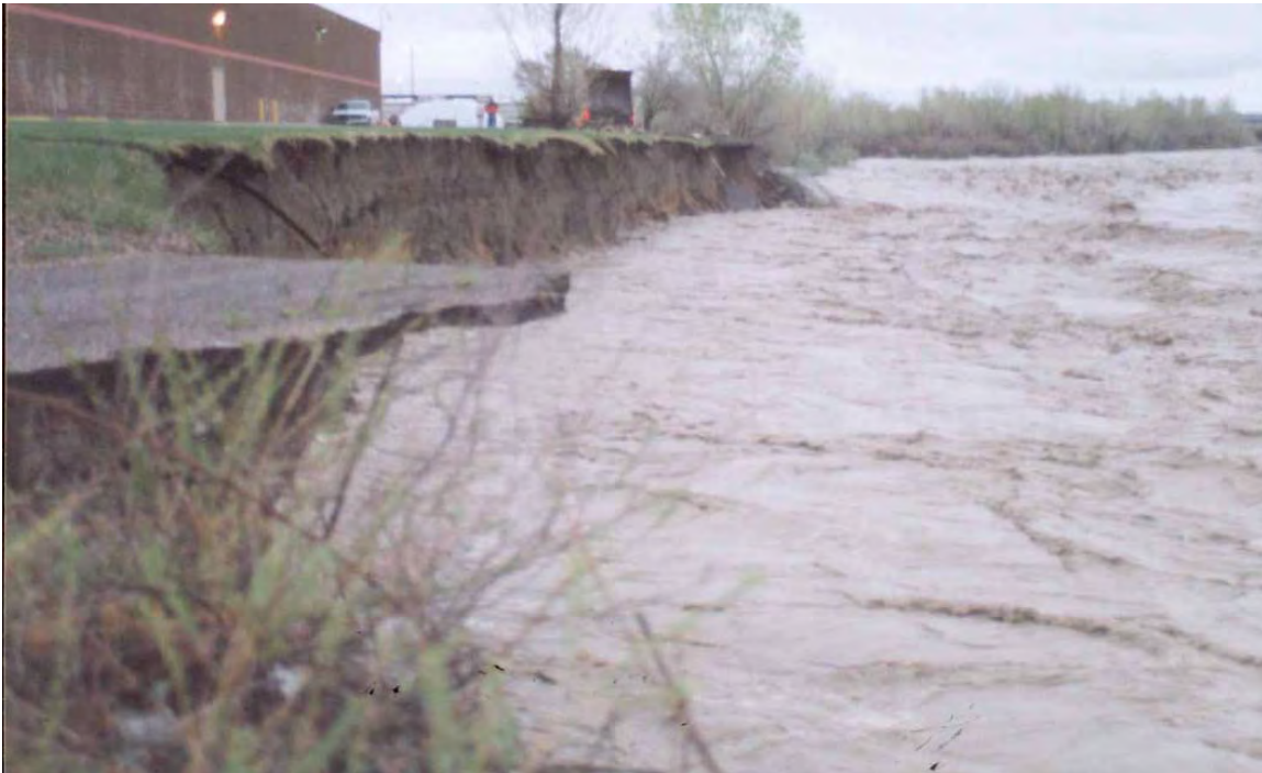
Photo 1-13. Erosion at the Target store in Pueblo during the 1999 flood.
