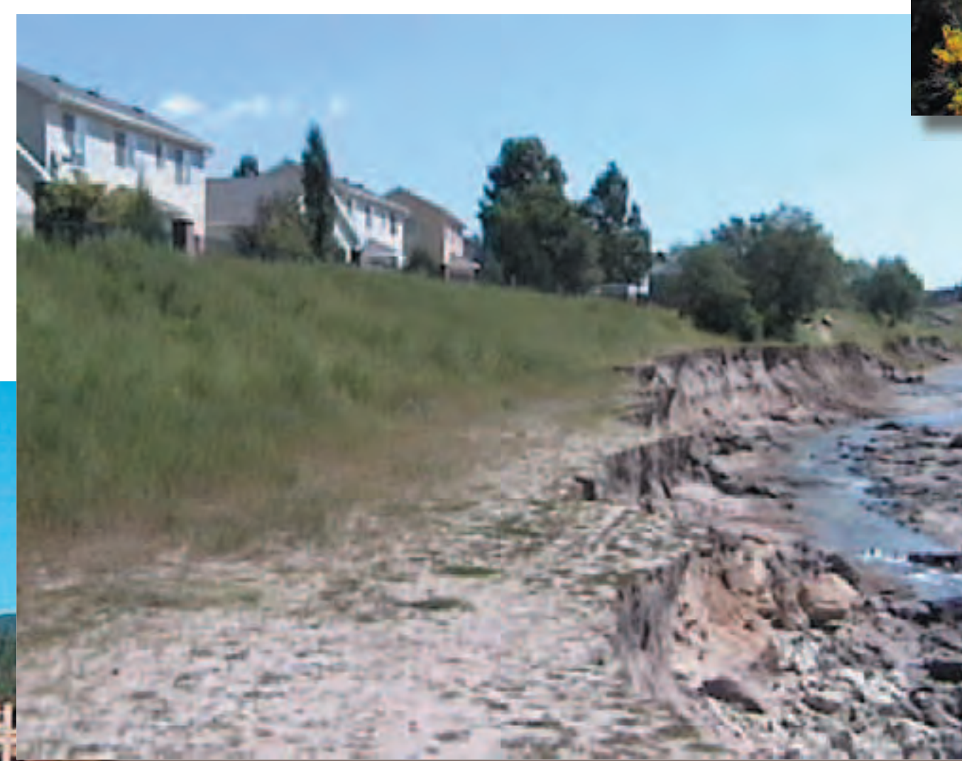
Cottonwood Creek Bank Erosion
