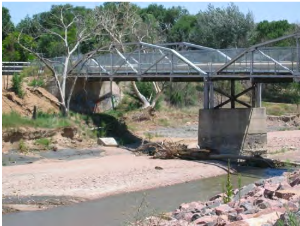
Photo 2-3. Fountain Creek at USGS Security Gauge Downstream view of pipeline crossing showing evidence of degradation on bridge pier (0219)
