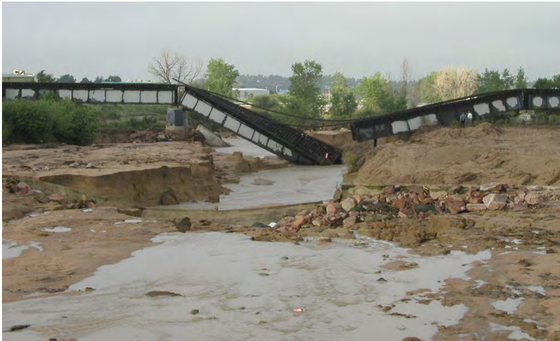
Photo 1-16. Erosion in Sand Creek immediately downstream of Sand Creek Detention Pond 1.
