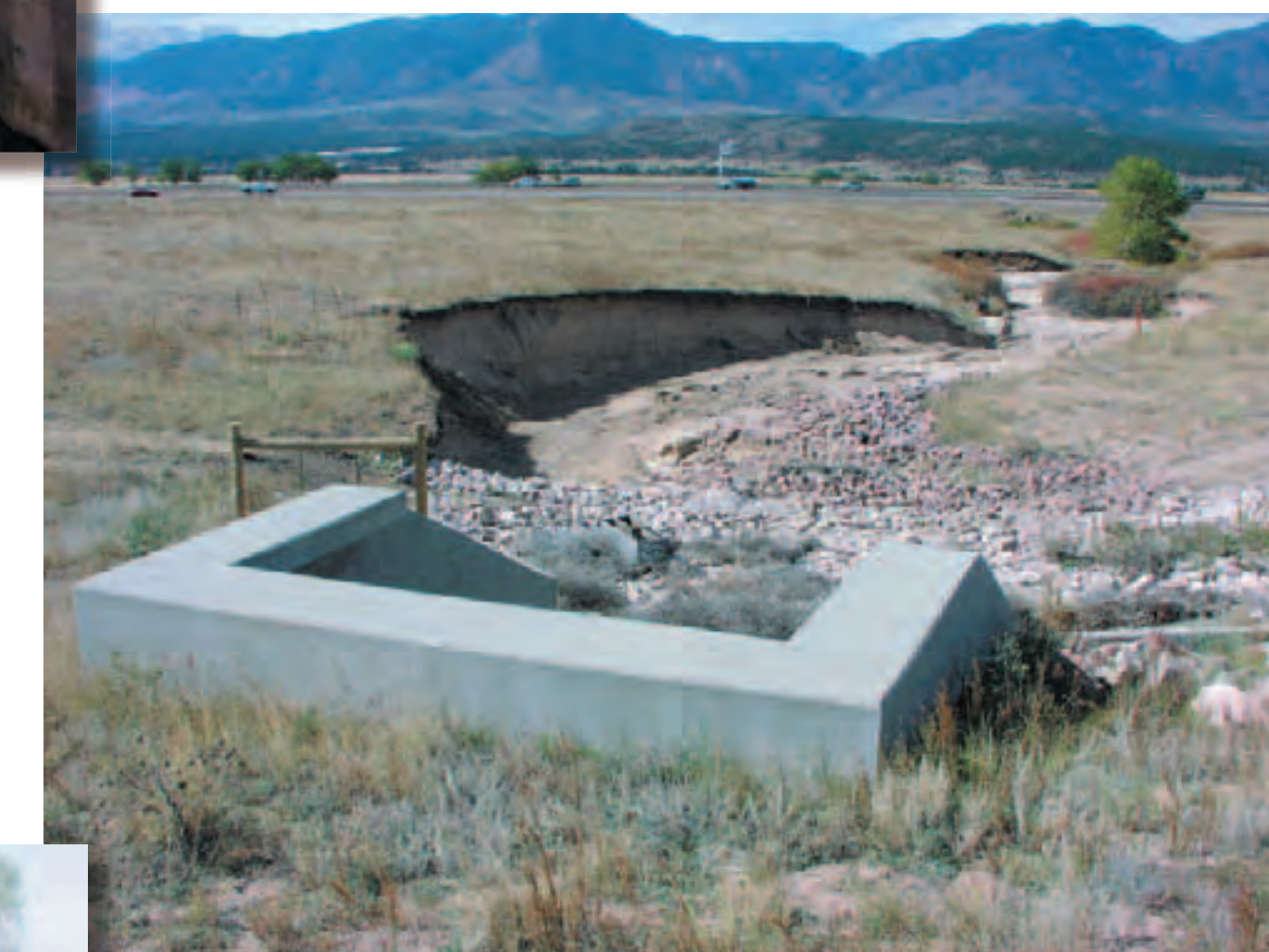
Erosion Downstream of a Detention Pond in the Elkhorn Basin
