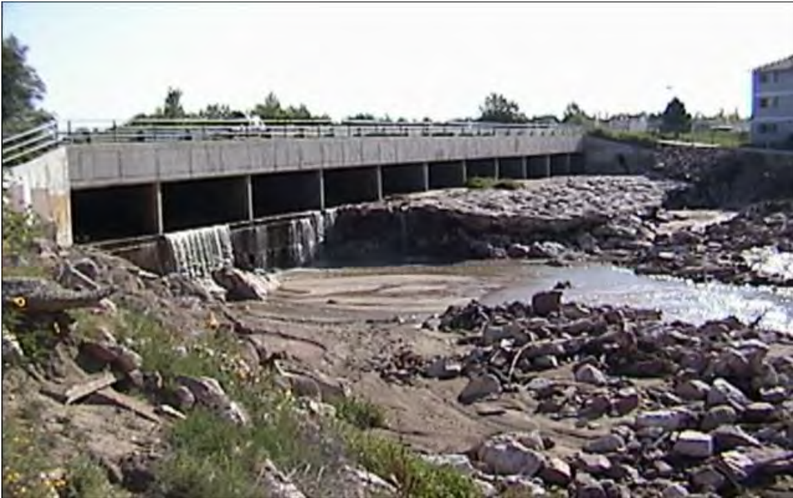
Photo 1-7. Erosion on Sand Creek below Chelton Road in Colorado Springs.
