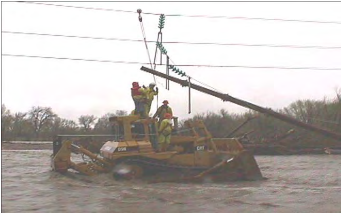
Photo 1-9. Damage to electrical utilities in Fountain.
