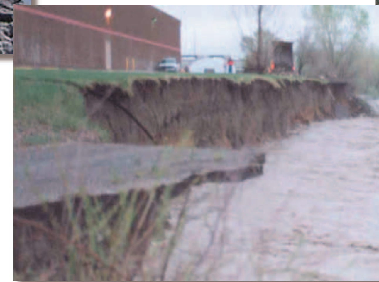
Bank Erosion in the Vicinity of Target Store in Pueblo
