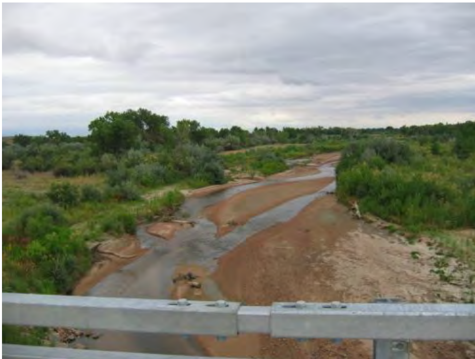
Photo 2-5. Fountain Creek at new Pinon Road Bridge Upstream view of typical channel reach with braided low flow (0367)
