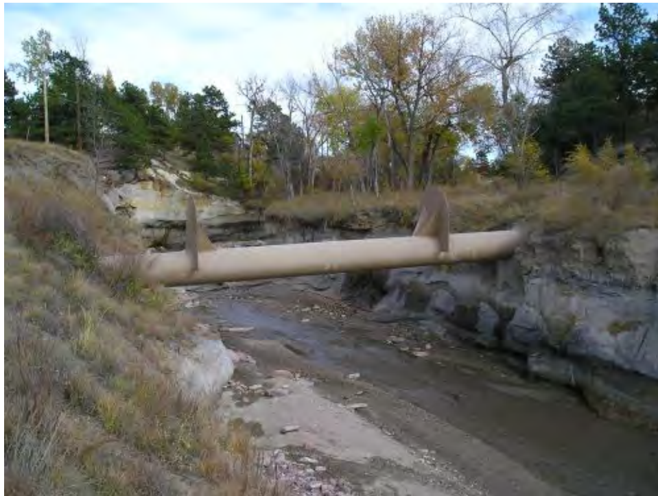
Photo 2-12. Cottonwood Creek near Wicklow Circle Upstream view of a suspended utility and severe channel degradation (0693)
