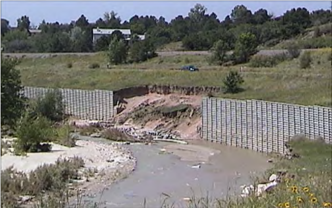
Photo 1-5. Damage on Monument Creek in Colorado Springs.
