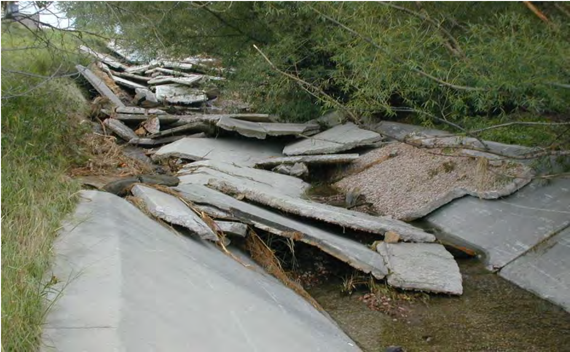
Photo 1-6. Damage at Rampart Park in Colorado Springs.
