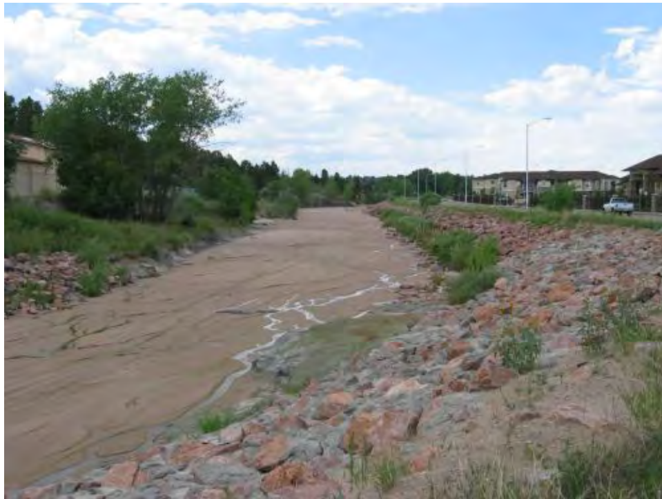
Photo 2-16. Sand Creek along Space Center Drive Upstream view of channelized reach in Sand Creek; riprap on banks (0296)
