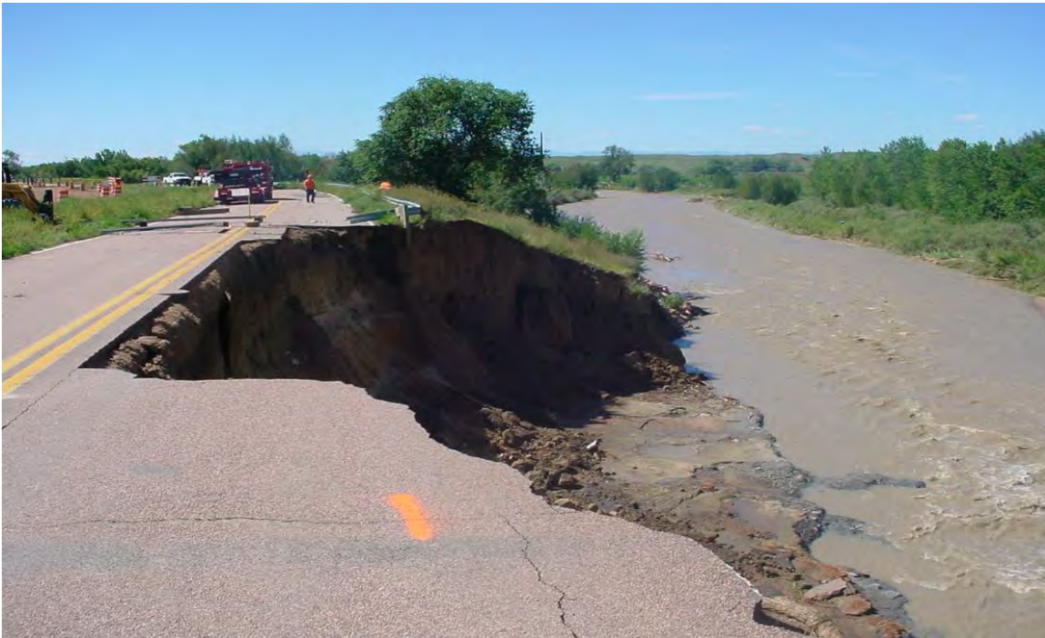
Photo 1-11. Erosion at Old Pueblo Road in El Paso County.
