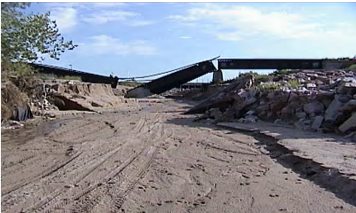
Photo 1-4. Collapsed Railroad Bridge on Sand Creek.
